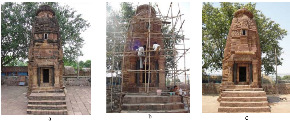
Fig. 4. Sita Devi Temple front view with stairs: a - before conservation; b – during conservation, c – after conservation
