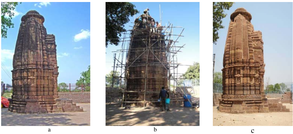
Fig. 3. Sita Devi Temple lateral view: a - before conservation; b – during conservation, c – after conservation
