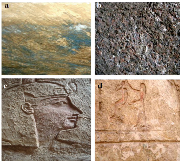
Fig. 1. Isolation of yeast strains: Samples were taken from (a) azurite blue on the ceiling of the tomb of Oserkon II , (b) granite blocks in the tomb of Psunis with a high humidity and microorganisms, (c) the eastern wall of the tomb of Oserkon II , (d) the red pigment from the tomb of Shashanq III .
