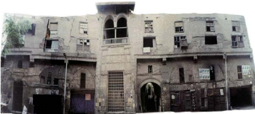
Fig. 7. Rabaa, Kutab and Sabeel Al-Qazzlar in Cairo. Before restoration and intervention processes
