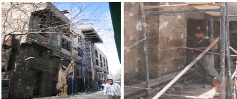
Fig. 8. Rabaa, Kutab and Sabeel Al-Qazzlar in Cairo. During restoration and intervention processes
