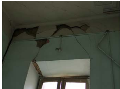
Fig. 11. Cracking at openings' corners
