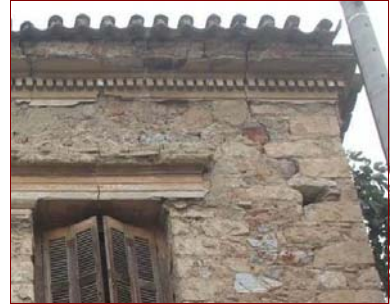
Fig. 9. Vertical cracking at to edge (crowning) of the façade of the building
