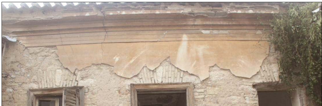
Fig. 12. Loss of plaster revealing mortar fragmentation (bleeding)
