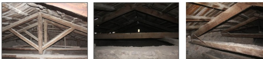
Fig. 6. Truss of central (left and right) and wing (middle) parts of the roof
