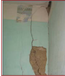
Fig. 8. Near vertical cracking of walls near their joint and splitting of wall-to-wall joint
