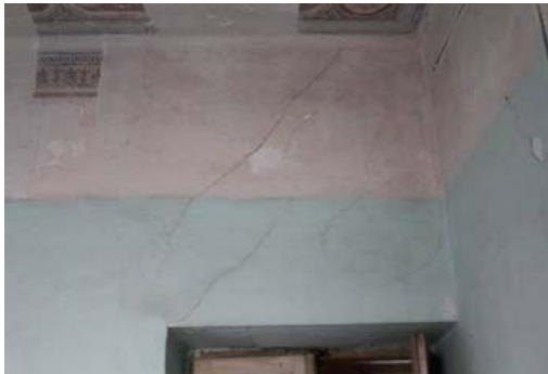
Fig. 10. Inclined splitting of masonry wall
