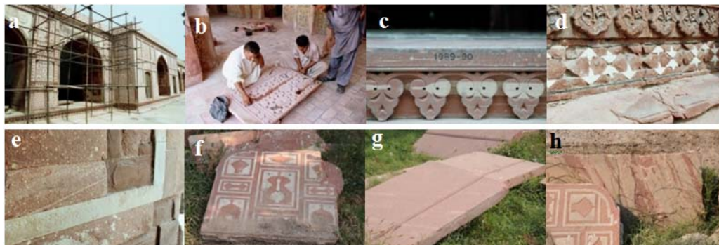
Fig. 1. Mughal Sandstones Heritage showing; a) Jahangir tomb rear façade under restoration, b) newly carved sandstone slab ready for inlay works, c) sandstone slab replaced in 1989-90 with elongated flattened whitish spots, d) deteriorated siltstone dado slab, e) yellow coloured sandstone used geometrically with red coloured sandstone, f) sandstone slab used during Mughal period, g) sandstone slabs imported from India after partition for restoration and h) Khewra/Sargodha sandstone
