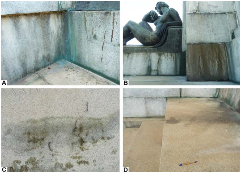
Fig. 5. Standards for the soiling found on the Monument to Ramos de Azevedo.
