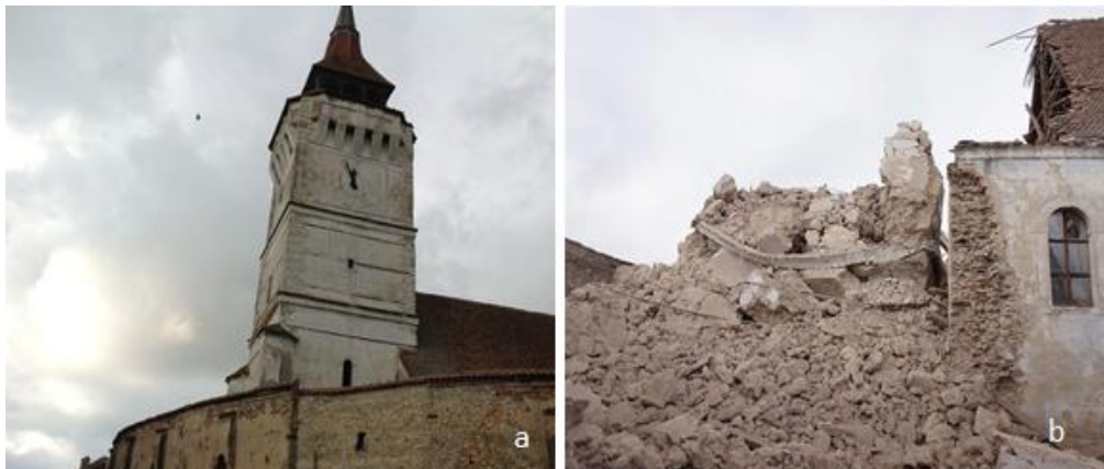
Fig. 8. The Tower of the Evangelical Fortified Church, Rotbav , Brasov: a. The church tower before collapse; b. The church tower after collapse [Photo source: a. Țetcu Mircea Rareș , 2013; b. http://tinyurl.com/j5tre9g ]
