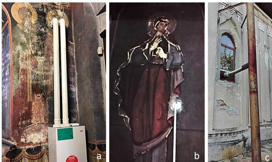
Fig. 6. Inadequate installation of heat and power systems inside of the historical monuments:
