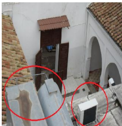
Fig. 10. Air conditioning units and water tanks on the mosque terrace
