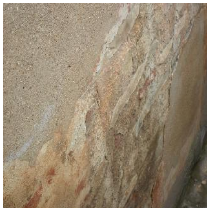
Fig. 8. Detachment of cement coating
