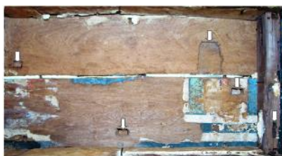
Fig. 7. Numerous of old mortises and remains of painted drawings in roof and cornice, shrine GEM_No 21072
