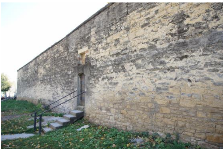
Fig. 4. Presence of black crust in North part of the perimeter wall of Galata Monastery (note: the respective crust also affected the lithic framing of a secondary pathway)
