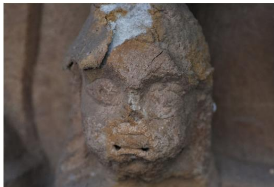
Fig. 3. Particular of a capital. Losing of the carving due to the action of the ageing of a synthetic adhesive applied in a previous restoration.
