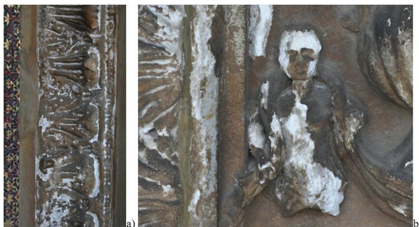
Fig. 2. Particular of piers: a) state of conservation of the marble with salts efflorescence, sugaring, powdering, black crust, browning of the surface due to the previous covering; b) losing of the flourishing shape due to the effect of the salts efflorescence with following sugaring and powdering of the marble.
