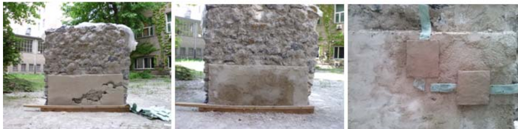
Fig. 2. Lacunae in the arriccio of the testing masonry. The plaster was applied only in the lower portion of the wall (a). After the mapping, the lacunae were covered with a thin layer of plaster sustained by a tissue (b). Detachment of the finishing layer (c).
